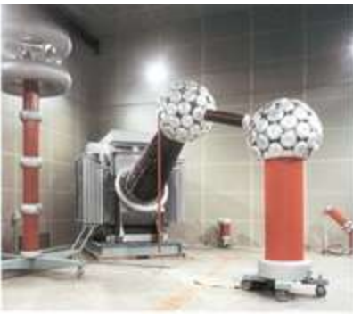
Segmented electrodes(Complete HV lab (600 kV AC))
